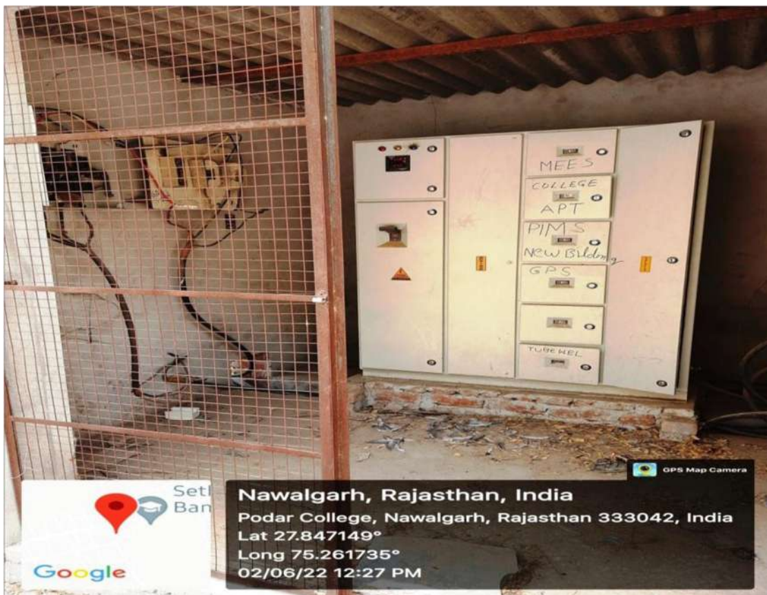
Electric Power Room
