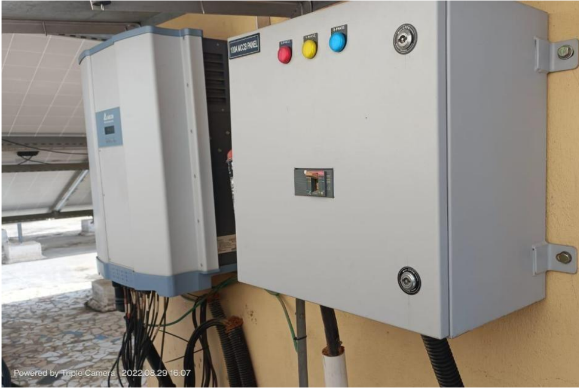
Solar Energy System
