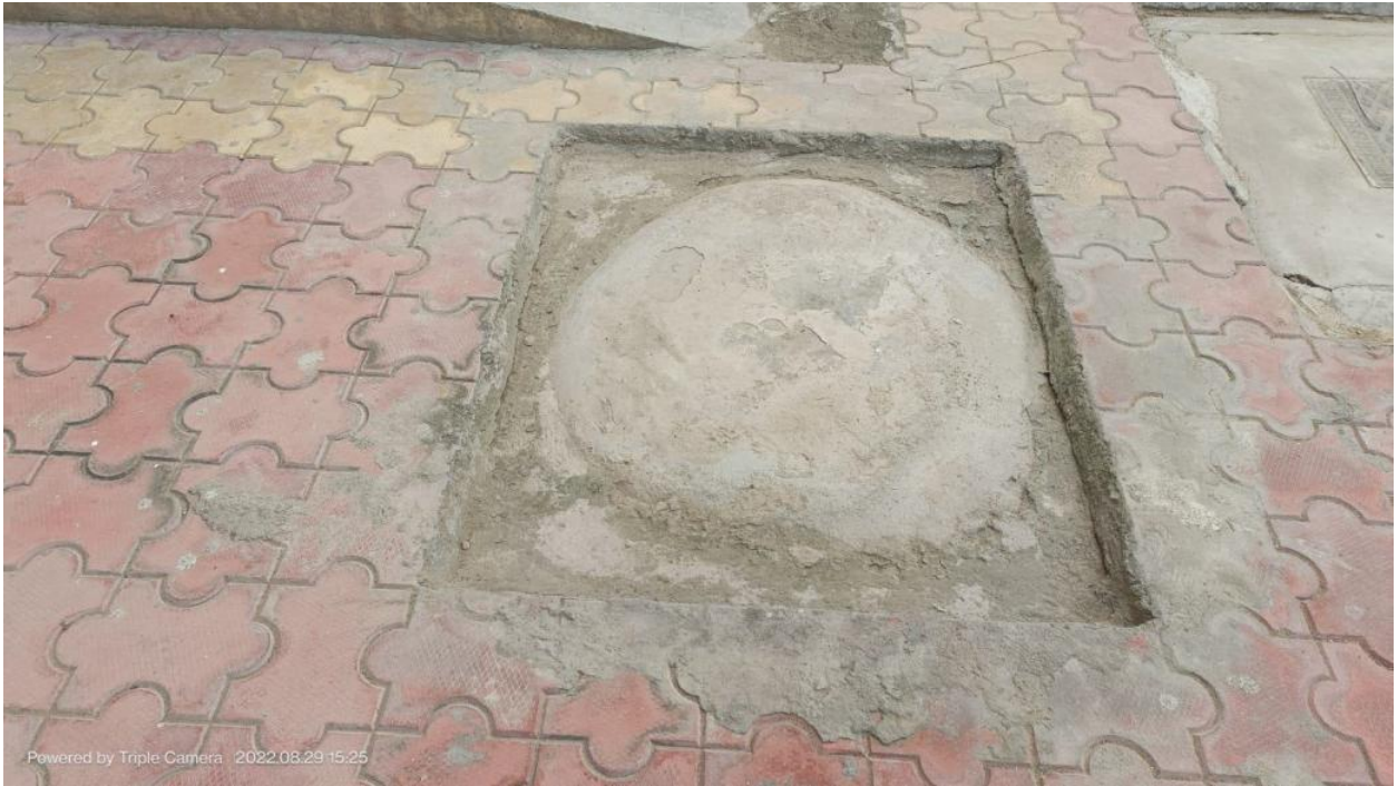
Safety Tank of Toilets
