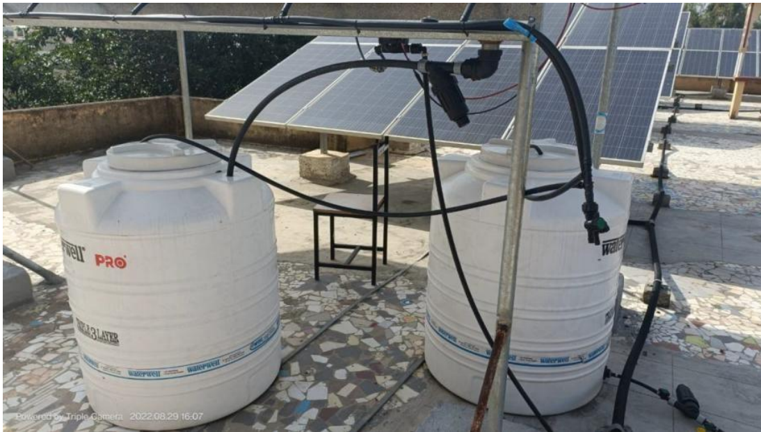
Water Purification System with Solar Energy System
