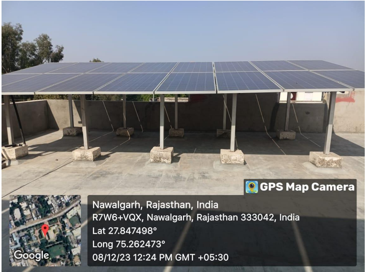
Solar Energy System in the PIMS Block
