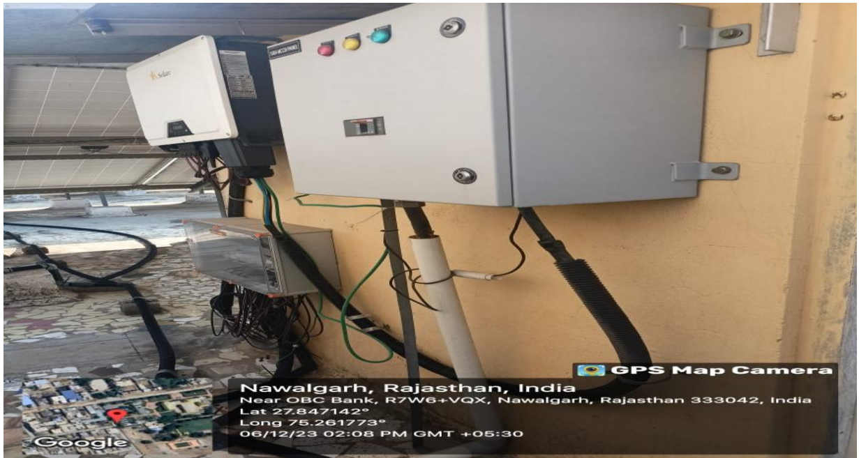
Solar Energy System in the PIMS Block
