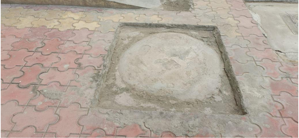
Safety Tank of Toilets
