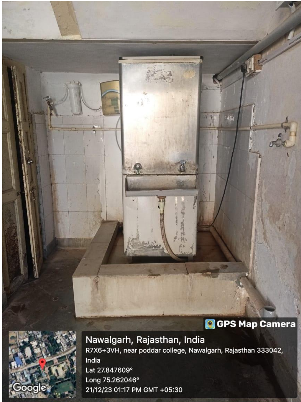
Water cooler Facility in PIMS Block
