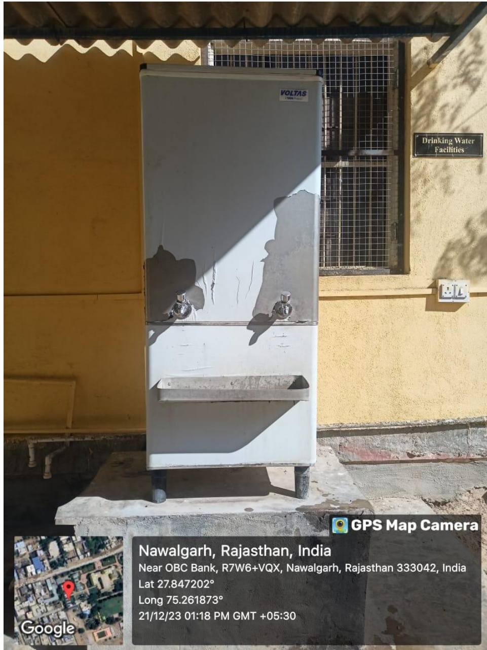
Water cooler Facility in Arts and commerce Block
