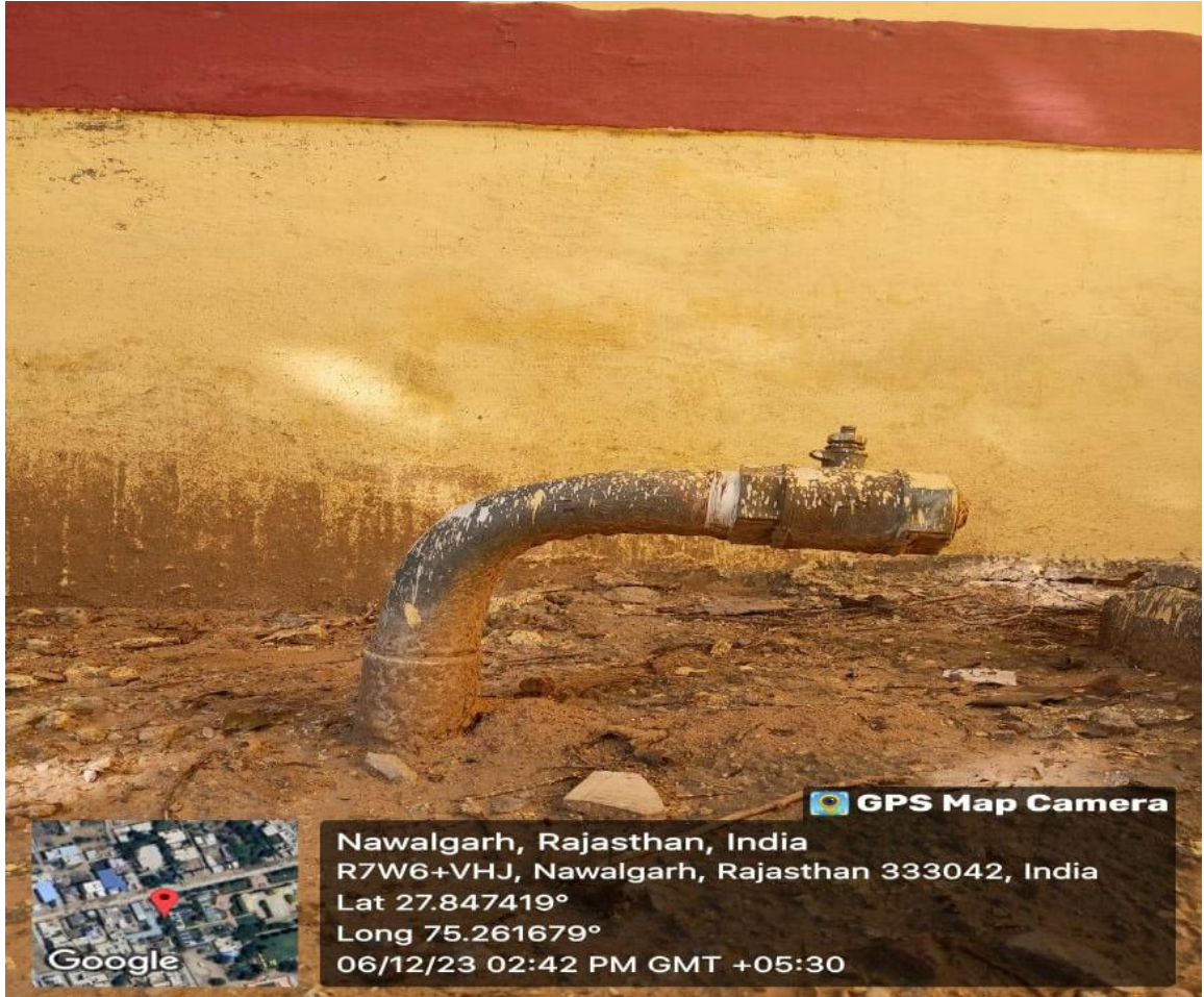
Bore well point in the Arts and Commerce Block
