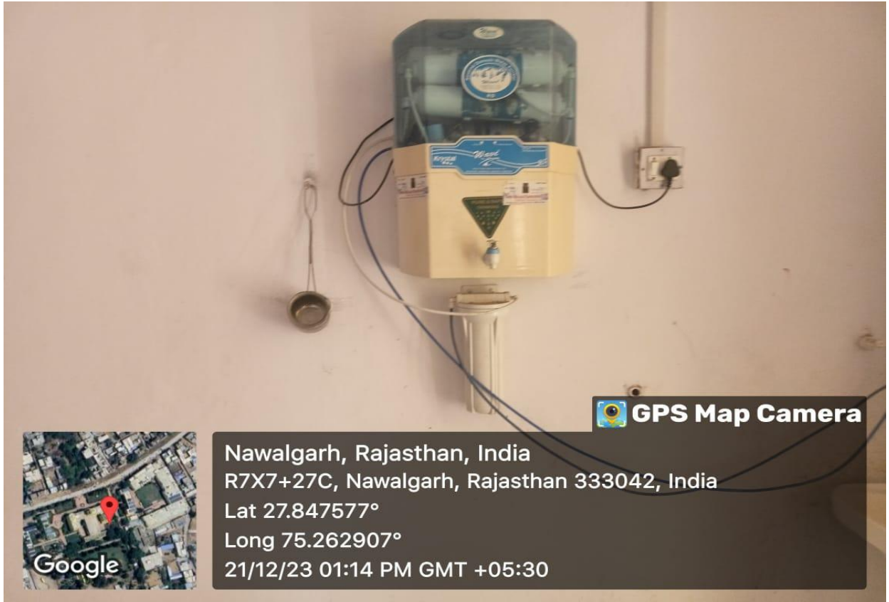
RO Water Facility in girls' common room
