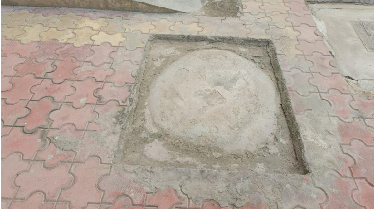
Safety Tank of Toilets
