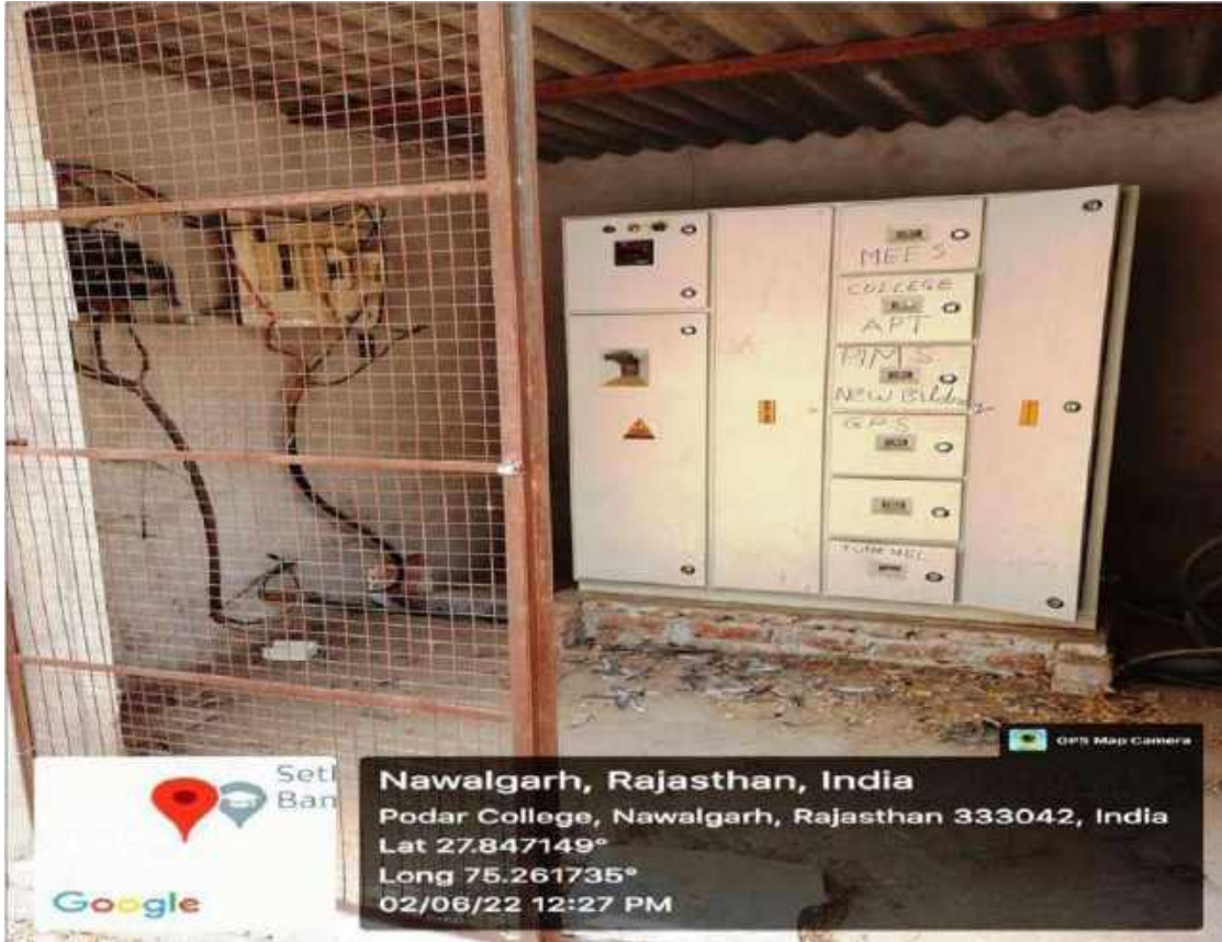
Electric Power Room
